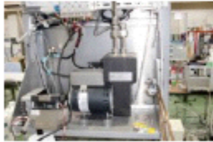
pump of the gas circulation
