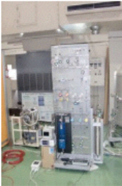
Control system of cryogenics
